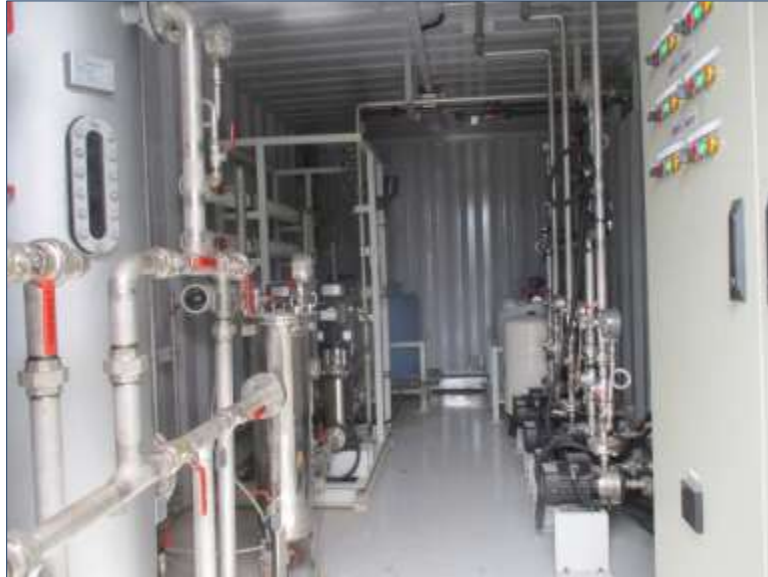
Reverse Osmosis House Unit 1 Interior View
