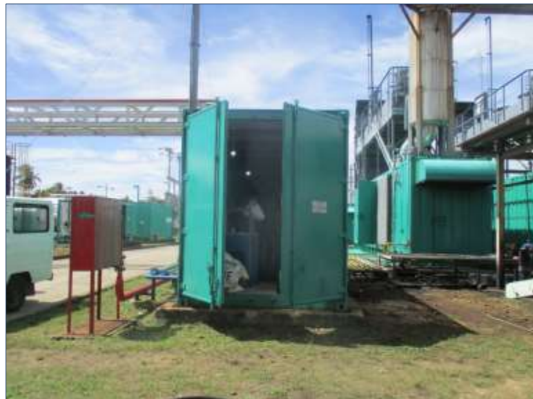
Air Compressor House
