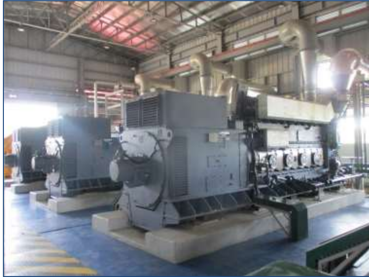
Powerhouse Interior View
