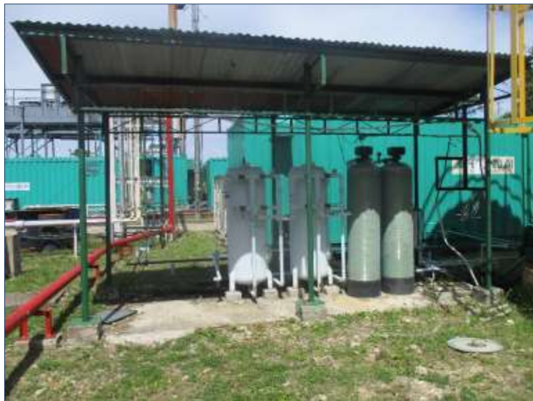
Water Softener Shed
