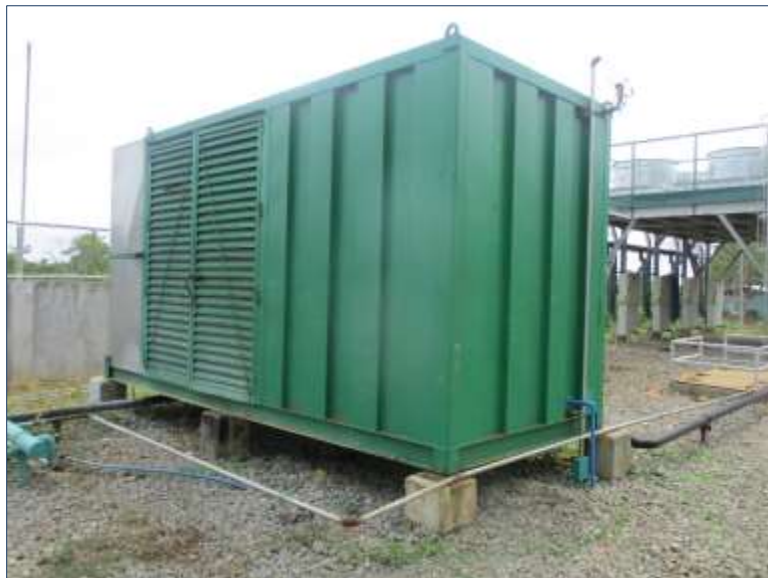
Reverse Osmosis House Unit 2
