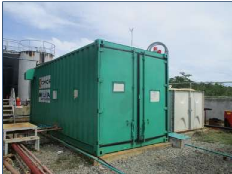
Reverse Osmosis House Unit 1
