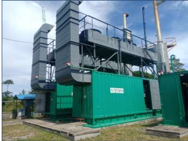
Diesel Power Generators
