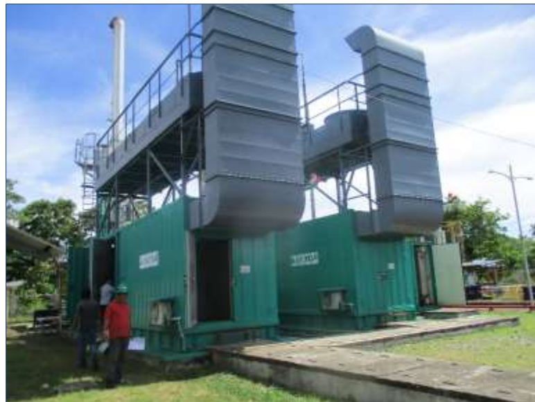
Main Diesel Unit House (2 Units)
