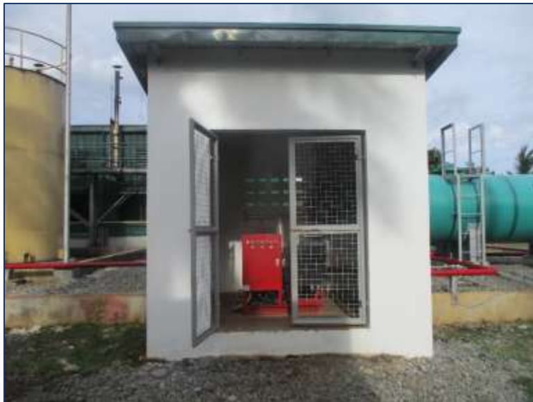
Fire Pump House
