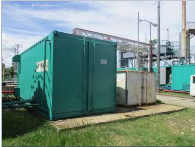
Water Treatment Unit House
