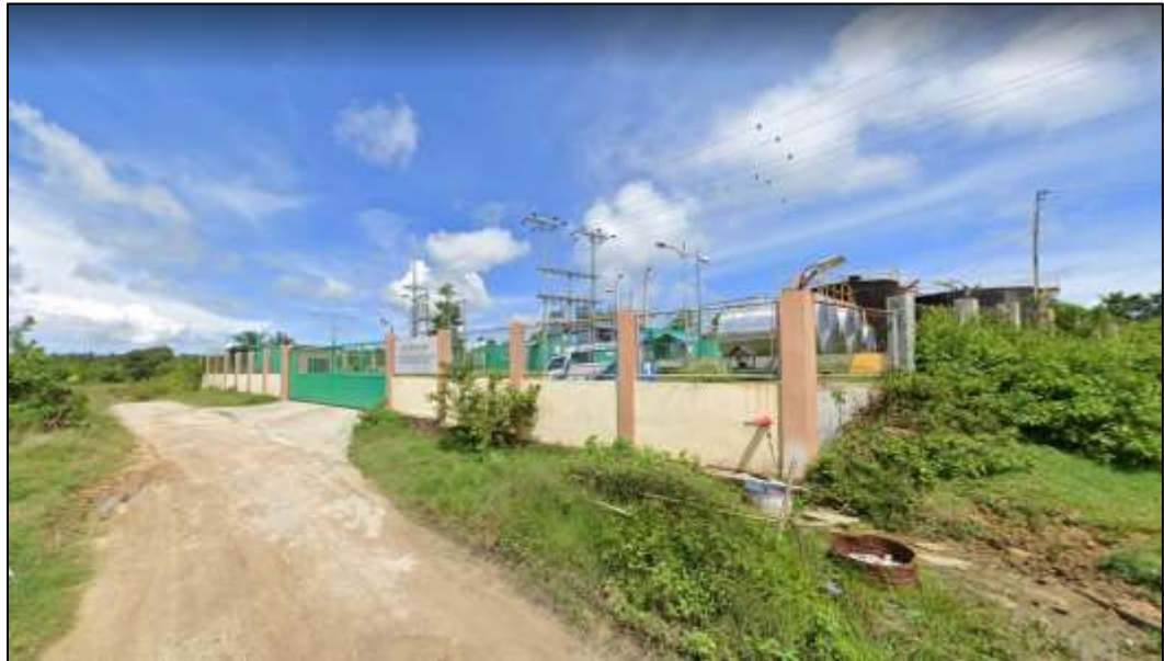
Figure 3: Siquijor Island Power Corporation (SIPCOR) 1 - Lazi
