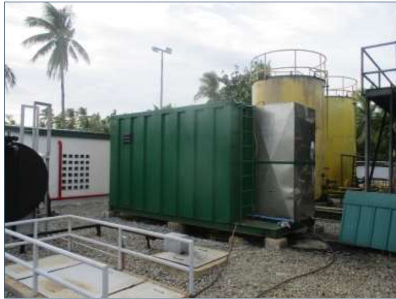
Reverse Osmosis House Unit 1
