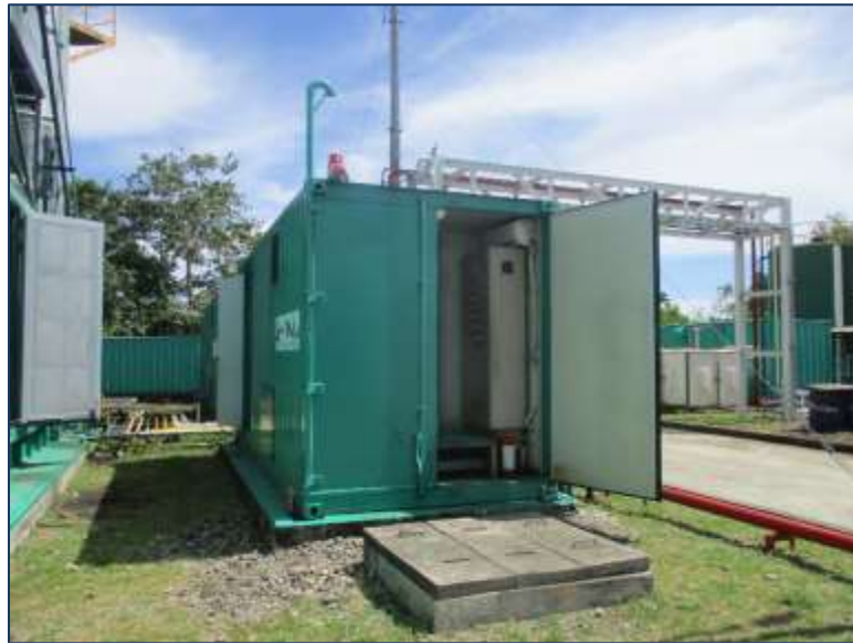
HFO Treatment Unit (HTU) House
