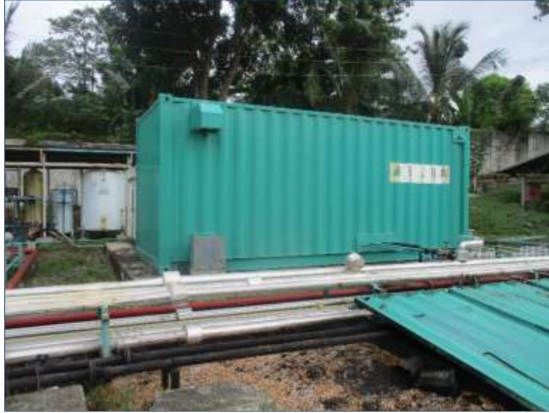
Water Treatment Unit House
