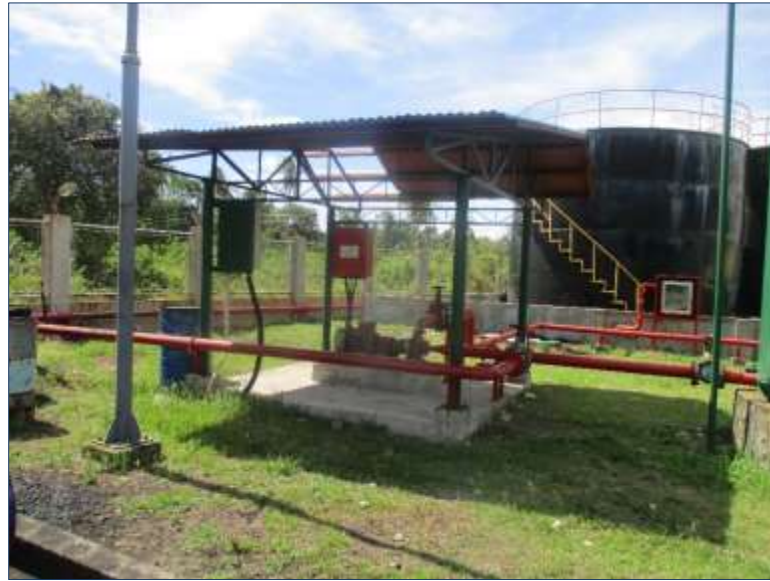
Fire Pump Shed
