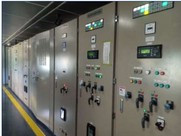
Medium Voltage Switchgear
