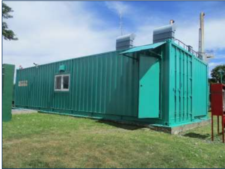
Control Room (Electrical Unit)
